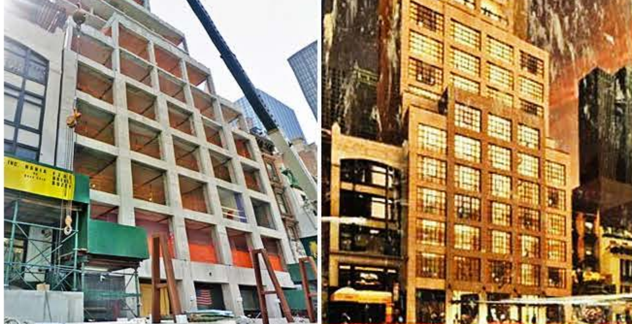
Construction underway at 18 W. 56th St., the future site of the Whitby Hotel; inset: Rendering of the hotel (Inset photo: New York Yimby)
